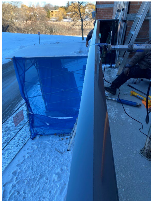
Photograph No. 8 Handrail Mid-Section Outward Load Deflection
